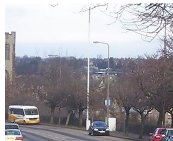
Figure 3: A 'micro-cell' base-station (which appears like another street lamp)
